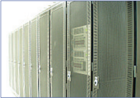
Secure, individually locked, 48U Cabinets house and protect customer owned hardware.
